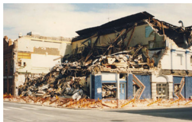
The impact to the RSL Club building, Newcastle. Source: Telstra Museum, Newcastle
