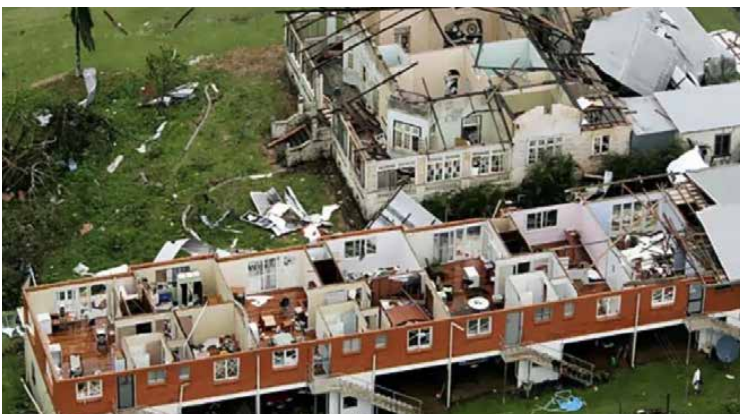
Figure 28: Houses and apartment blocks with their roofs blown off in Innisfail after Cyclone Larry struck in March 2006. Source: Mark Baker(AP)
