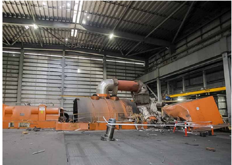
Figure 106: Damage to Unit C4 at Callide Power Station following the plant fire on 25 May, 2021. Source: CS Energy.
