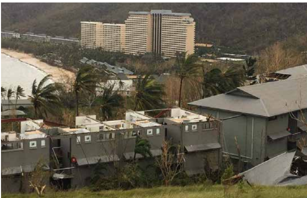
Figure 54: Roof damage sustained to holiday accommodation on Hamilton Island. Source: ABC News (Dennis Garrett)
