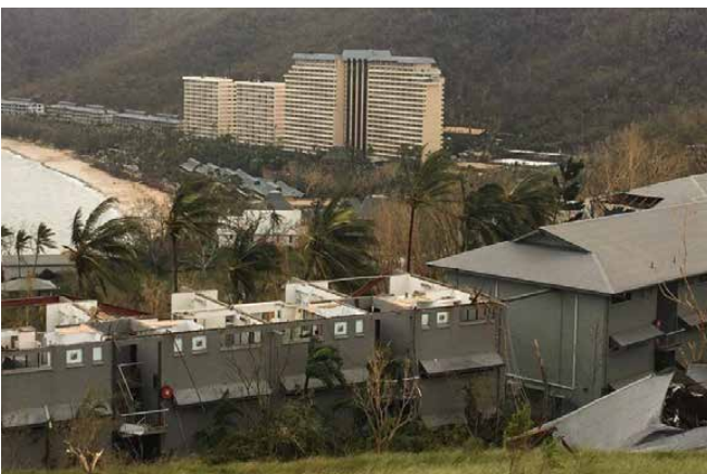
Figure 35: Roof damage sustained to holiday accommodation on Hamilton Island from Cyclone Debbie. Source: Dennis Garrett (ABC News)
