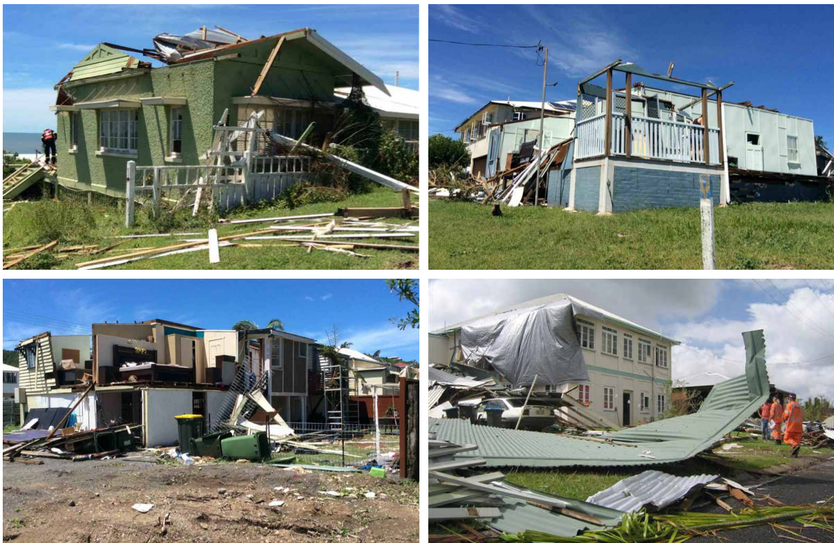
Figure 51: Damage to buildings in Yeppoon in the aftermath of Cyclone Marcia, 2015. Source: Queensland Fire and Emergency Services
