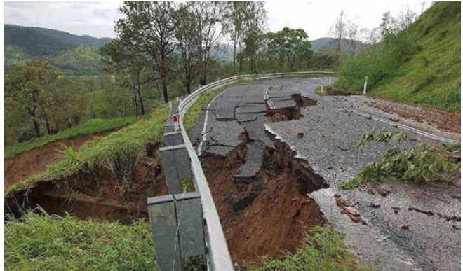
Figure 33: Serious damage around Sarina Range due to landslips from Severe Cyclone Debbie. Source: Loretta MacGregor
