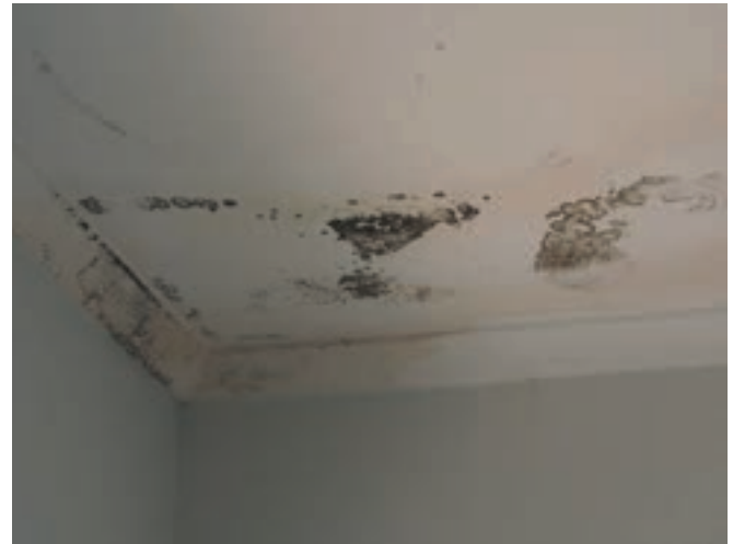
Mould on ceiling.
