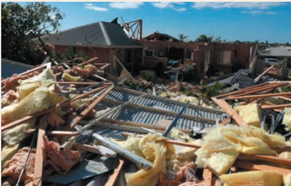
Figure 41: Damage to roof cladding and roof structure (CTS)
