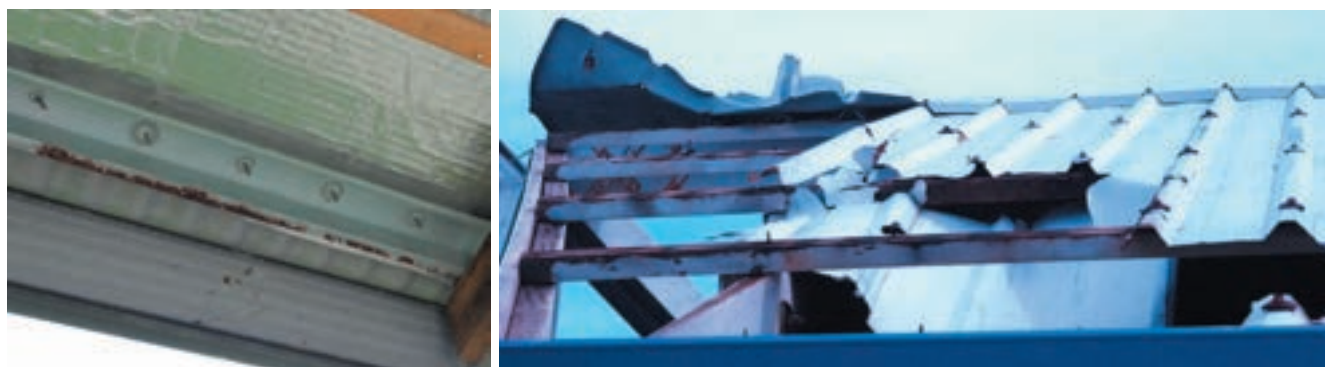
Figure 125: Examples of corroded battens and screws for properties near the coast. Source: CTS
