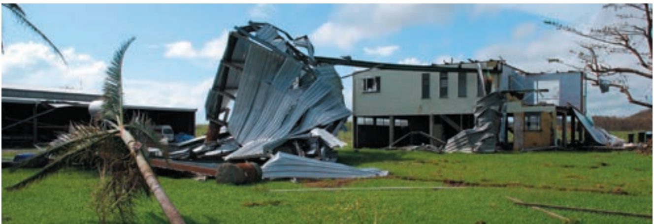
Figure 127: Very large wind-borne debris and the house it hit in TC Yasi.
