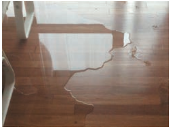
Water on timber floor.
