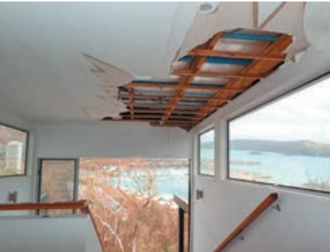
Damage to plasterboard ceiling from water ingress through the roof.
