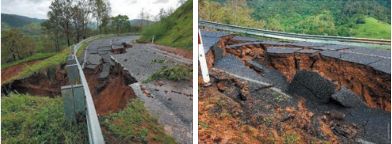
Figure 113: Serious damage around Sarina Range due to landslips from ex-TC Debbie. Source: Loretta MacGregor
