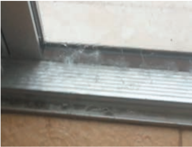
Rainwater bubbling through weep holes in windows.
