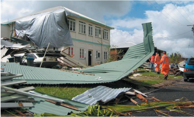
Figure 19: Damage to buildings in Yeppoon in the aftermath of TC Marcia, 2015. Source: QFES
