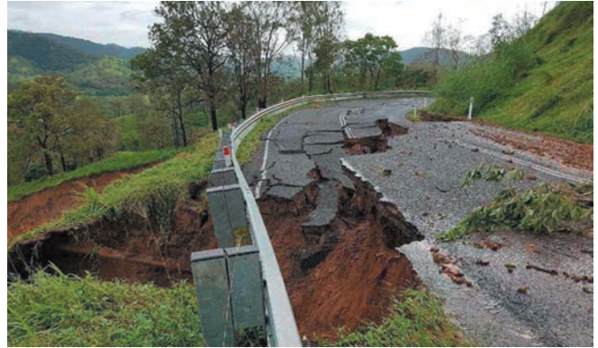
Figure 20: Serious damage around Sarina Range due to landslips from TC Debbie. Source: Loretta MacGregor
