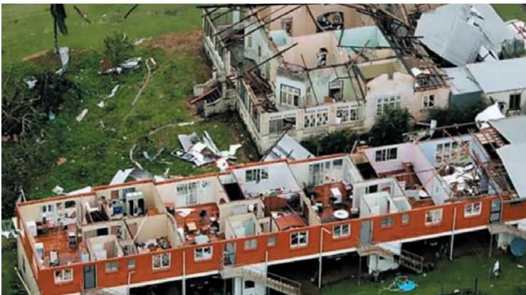
Figure 13: Houses and apartment blocks with their roofs blown off in Innisfail after TC Larry struck in March 2006. Source: Mark Baker(AP)
